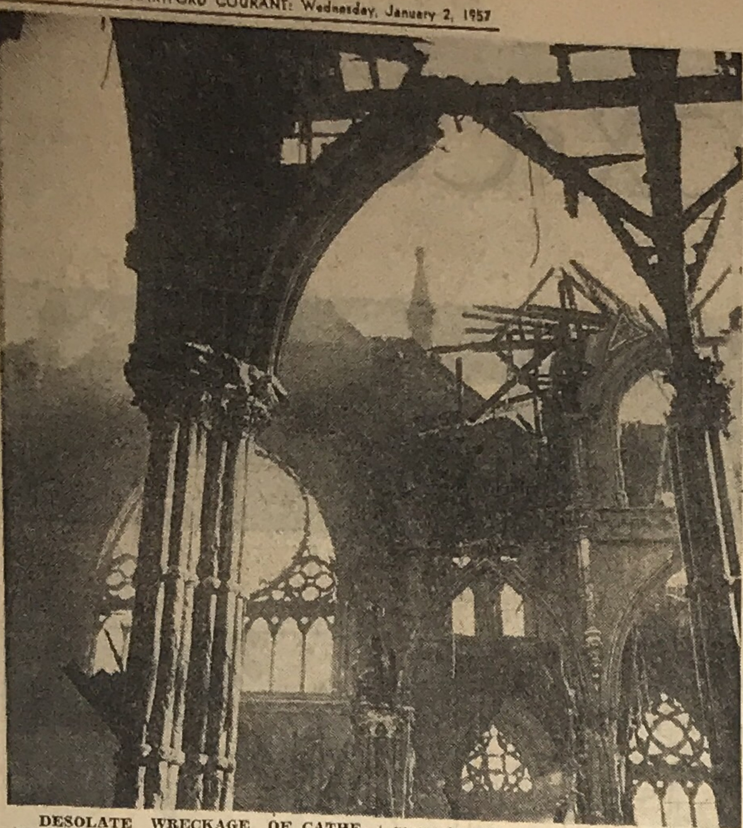
DESOLATE WRECKAGE OF CATHEDRAL: Blackened beams and empty windows present this stark appearance in St. Joseph Cathedral Tuesday morning. Many of the timbers seen ready to topple, making it too dan-
